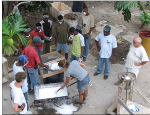
Slacking quicklime to create historic-grade lime mortar was one of the hands-on activities taught to students. The lime mortar will be used to repoint a late 18th century building. Jimmy Price of Virginia Lime Works is standing on the far right, and I am slacking the lime.
